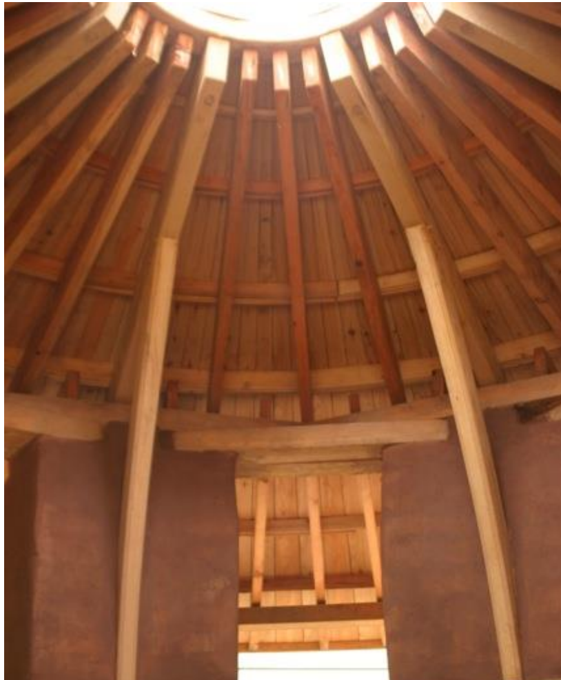
New outdoor cob classroom at Upton Cross Primary School. Works and photo courtesy of Clayworks.
